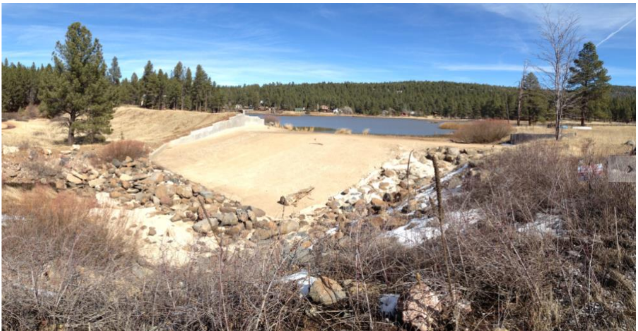
Figure 2: Current state of the dam's spillway.
